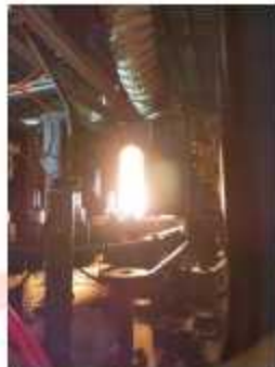
Gambar 11. Tampak samping heater . (Sumber : PT. Kiewell Plastik Packaging, 2022)
