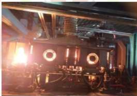
Gambar 12. Tampak belakang heater . (Sumber: PT. Kiewell Plastik Packaging, 2022)
