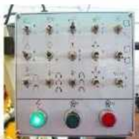
Gambar 7. Komponen Control Panel
